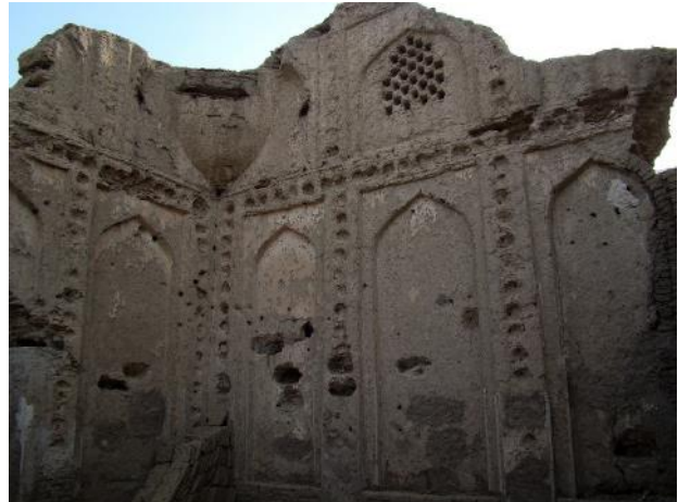
Figure 21. Inside of tomb no.1 Before restoration (Arcades and Squinch), (2010), (photo:M. Keyhanpoor)
